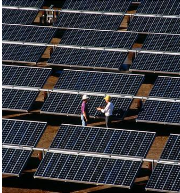
Figure 5.19-3. PV Panels in a Single-Axis Tracking System, Sacramento Municipal Utility District, Hedge Substation (Credit: Sacramento Municipal Utility District; Source: NREL 2009)
