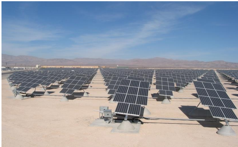
Figure 5.19-2. PV Panels in a Dual-Axis Tracking System, Nellis Air Force Base, Nevada (Credit: Argonne National Laboratory)
